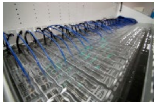
Figure 1. Server Racks and Chiller (Top) and Inside View of the Server Rack (Bottom) [1]
